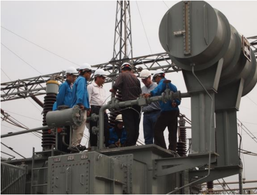
3.) Adjustment position of Motor Drive Unit (MDU) and OLTC before opening the transformer
