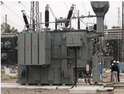
2.) Orientation around the transformer and it's components and preliminaries for OLTC inspection
