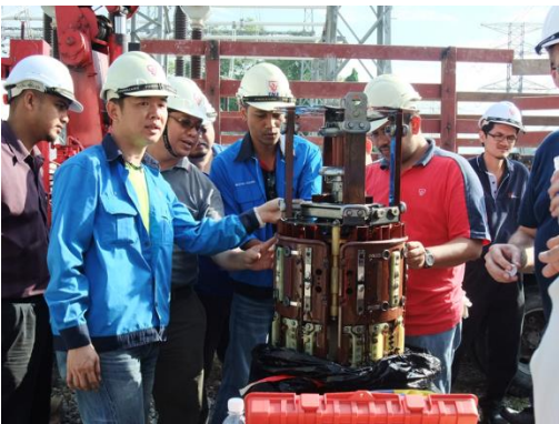
5.) Inspecting diverter switch by dismantling the support bars, energy accumulator and actuating system before removing the diverter switch contact shells to gain access to the moveable contact system
