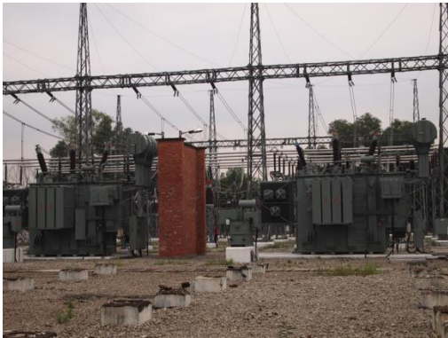
1.) Safety briefing (The participants have access to the top of the transformer (About 3.5 m high))
